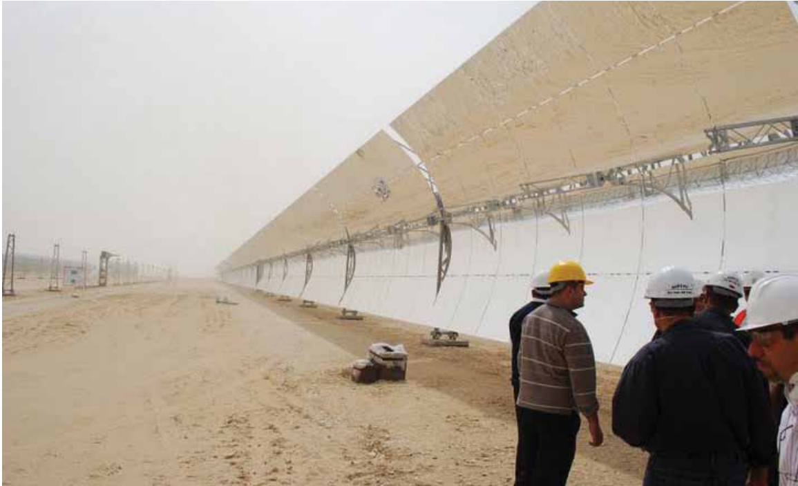
The WBG/GEF-financed Al-Kureimat solar thermal power plant in Egypt, under construction, March 2009.
